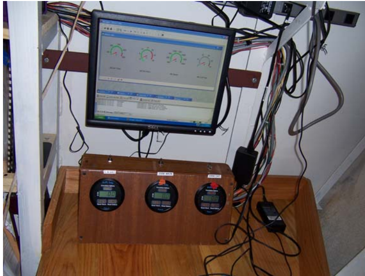
Figure 3: Engineer's station in bosun's locker of Blue Heron. Computer monitor displays the real-time measurements from the data acquisition system using dial indicators. Three gauges for monitoring the fuel consumption of the main engine and the two generators are located below the monitor.
