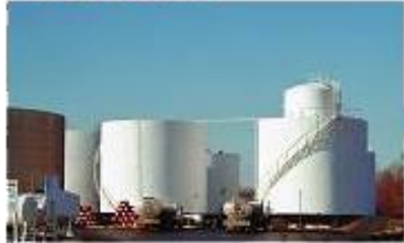
Diesel Fuel Storage at Refinery
