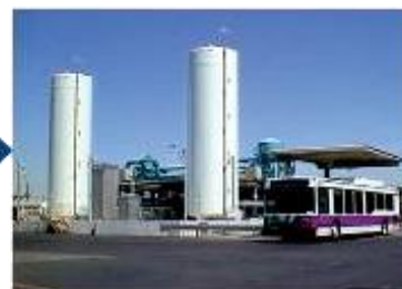
Above Ground Cryogenic Storage & Fueling Station
