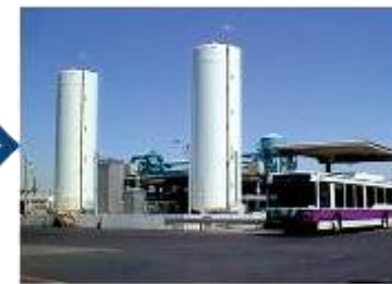
Above Ground Cryogenic Storage & Fueling Station
