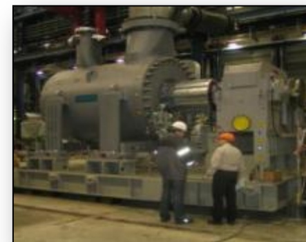
Photo courtesy of Siemens
