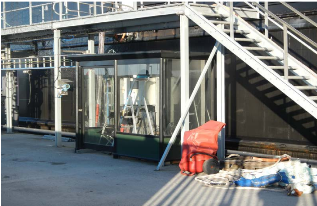
Figure 13 LNG Facility Cargo Control Area
