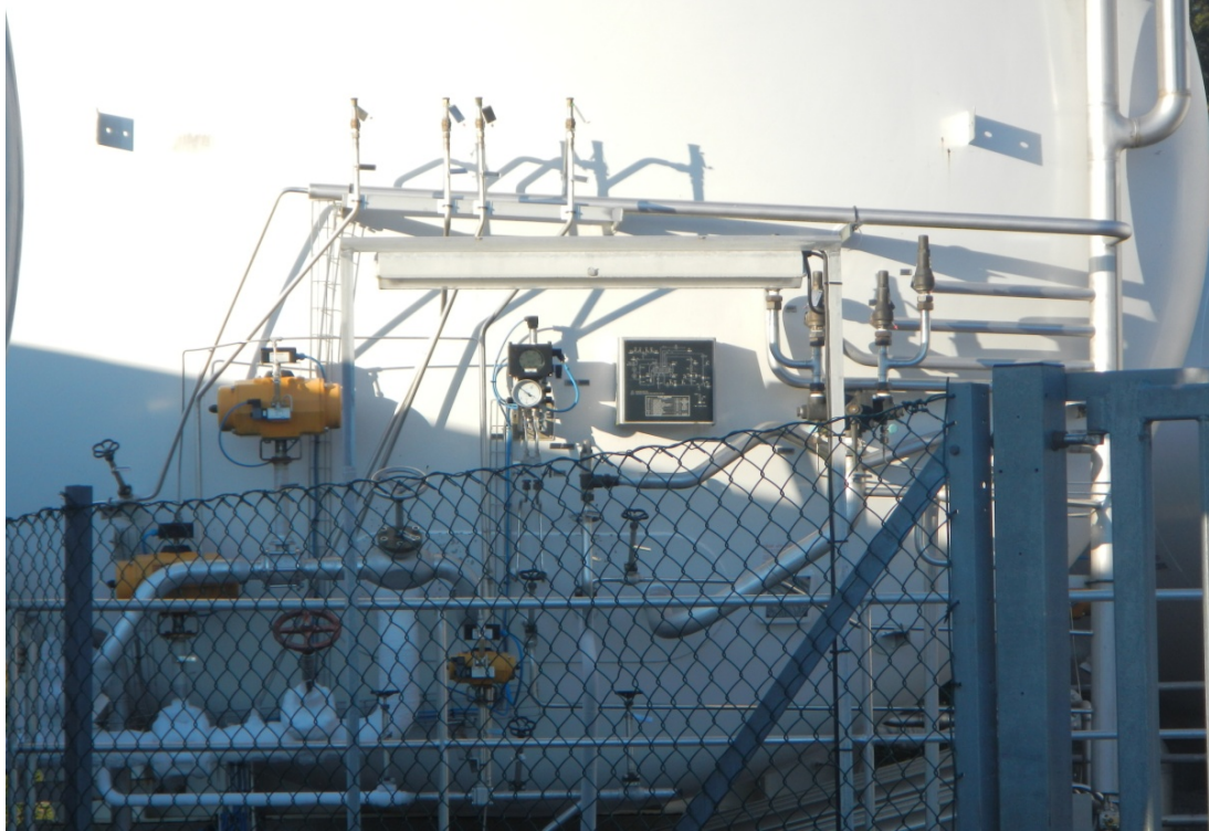
Figure 4 LNG Tank Gauges and Valves
