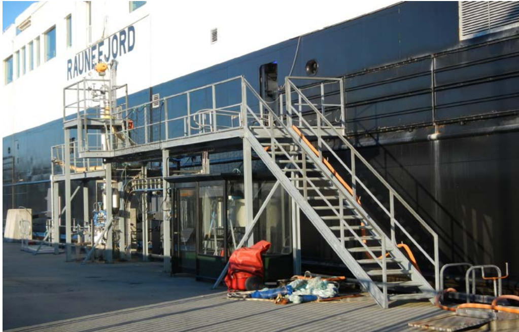
Figure 12 LNG Fixed Manifold and Piping
